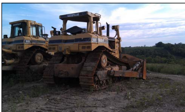
Bottom: Equipment ready to grade the property at the future Arcadia in Campbell County.
